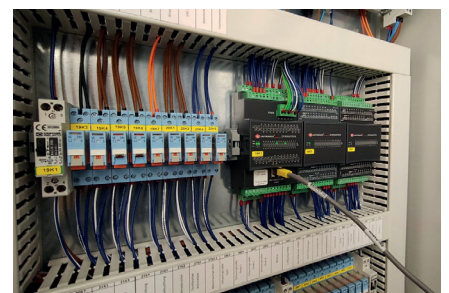
Control cabinet with PLC and ComatReleco products.
