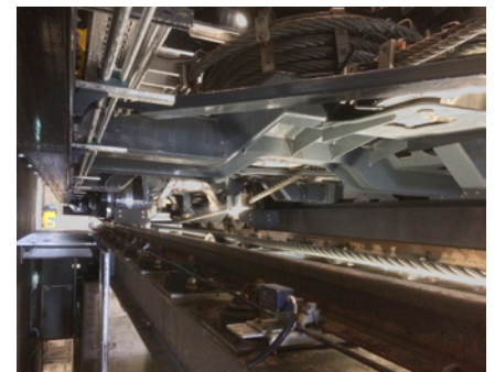
The electrical voltage of the funicular's hauling rope is measured at the valley station and compared with that of the mountain station. Deviations in the voltage stop the funicular.
